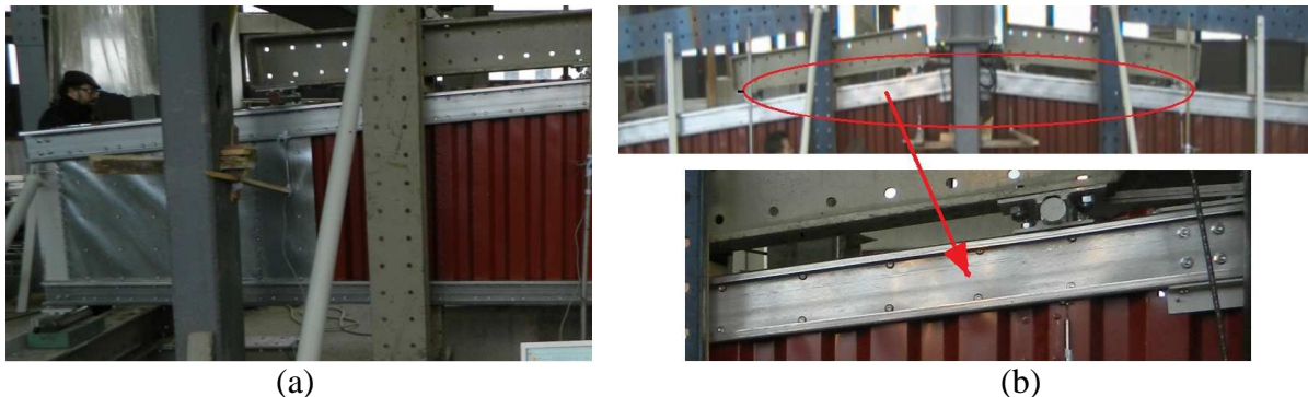
Fig. 9: (a) Deformed shape of the beam end shear panel; (b) local buckling of top flange
